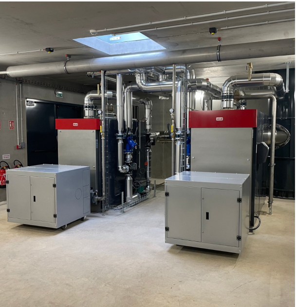
Varzy district heating network.
