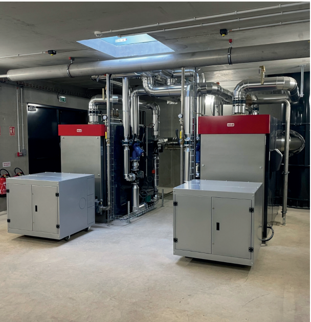
Varzy district heating network.
